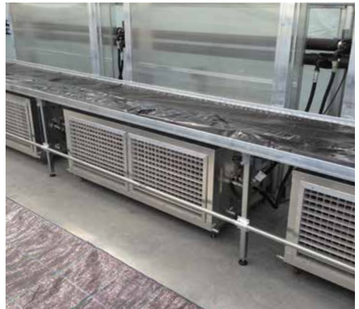
Chilled Water Fan Coil Units
