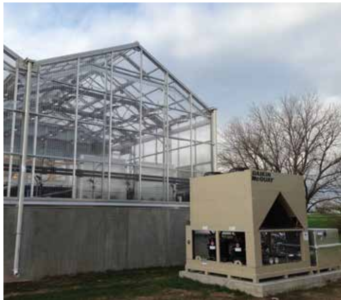
Chiller Pump Station
